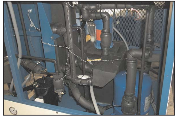
Interior View: The blue Maneurope compressor is located in the lower right. All plumbing is insulated with closed cell foam neoprene.
